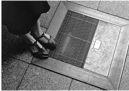
Figure 2. One of four ground grids with a loudspeaker and a light underneath the ground on the left side and two infrared distance sensors at the right side covered by a little window. Each loudspeaker cavity contains two sensors aimed in different directions.
